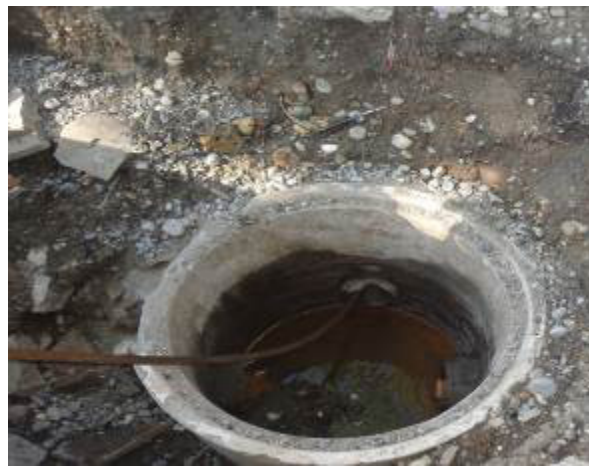
First the Ø 22 mm (0.86") pulling cable is slid through the old pipe.
