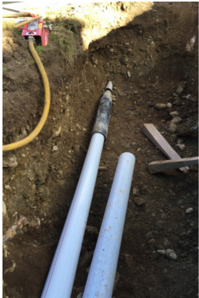
Picture 3: The new PE pipe OD 132 mm (5.2") is assembled into the expander. The expander drives the smaller pipe OD 92 mm (3.6") out of the pilot bore.
