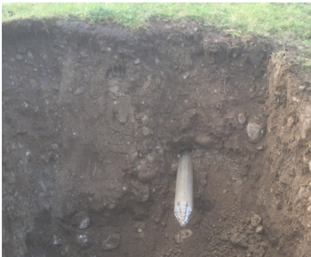
Picture 1: The TERRA-HAMMER T 105 S reaches the arrival pit right on target. The PE pipe OD 92 mm (3.6") is pulled in simultaneously. This avoids collapsing of the pilot bore.
