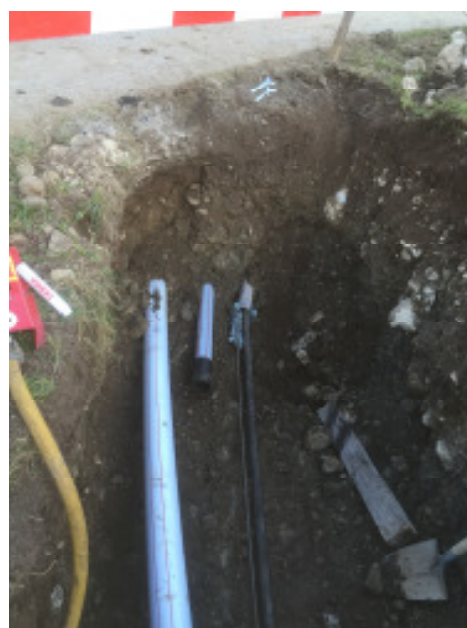
Picture 6: For this road crossing one PE pipe OD 132 mm (5.2") and two PE-pipes OD 92 mm (3.6") were pulled in.
