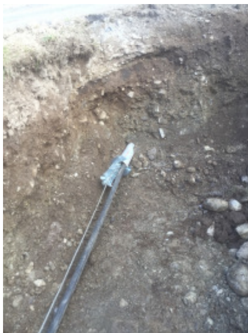
Picture 4: The cable clamp tensions the new PE pipe against the expander.
