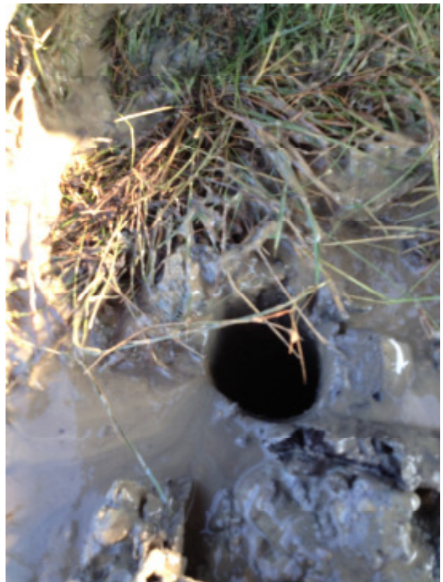
Picture 7: After 1 ½ hours 25 m (80 ft) at been drilled vertically. For the stabilisation of the bore hole \varnothing 100 mm (4"), 100 ltr/min (26 gpm) of Bentonite were pumped into the vertical bore hole.
