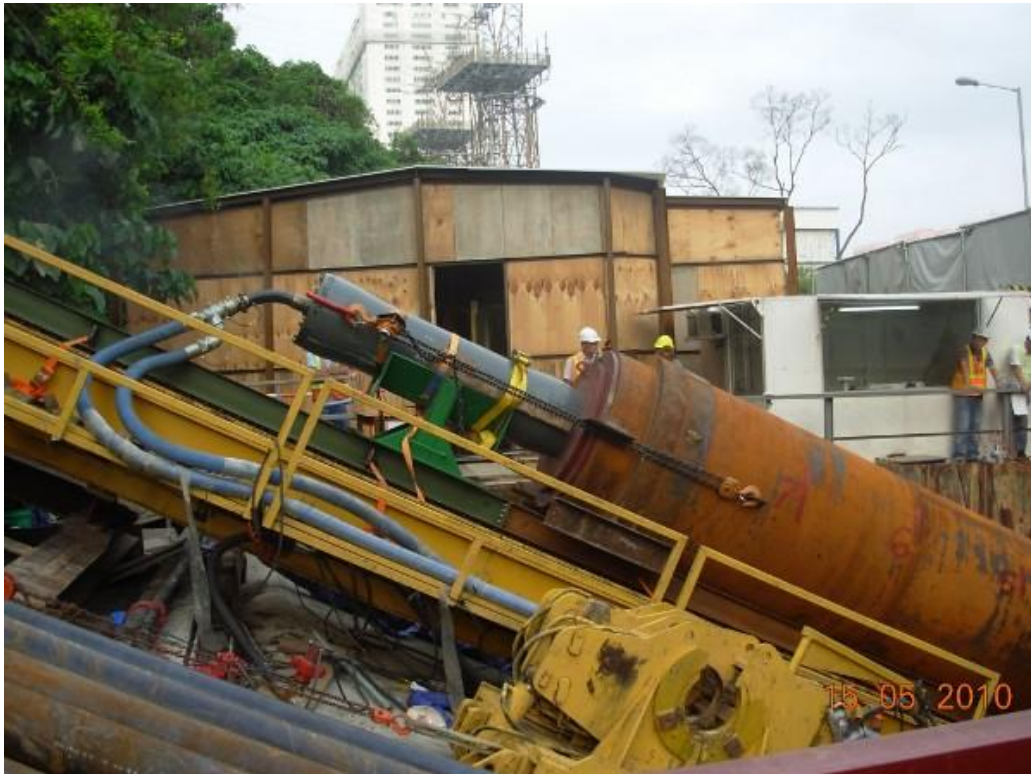
The TERRA-HAMMER TR 565 during the ramming of the steel pipe ø 1'400 mm (55")
